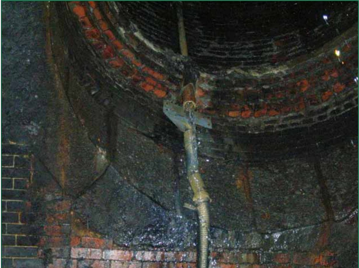
Figure 16: The broken downpipe in ventilation shaft 11
