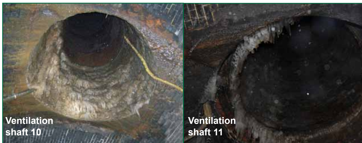
Figure 11: Views looking up at ventilation shafts 10 and 11 showing ice still present in the bottom of the shafts (ventilation shaft 11 photograph courtesy of British Transport Police)
