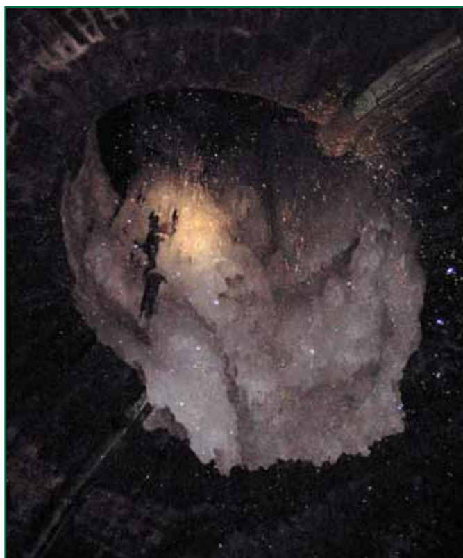
Figure 15: The ice formation seen hanging from the bottom of a ventilation shaft in Blea Moor tunnel in December 2010 (courtesy of Network Rail)
