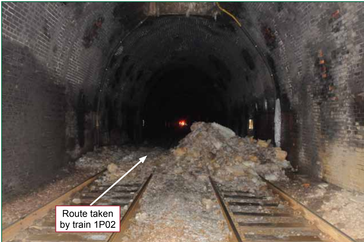
Figure 8: General view of the pile of ice found below ventilation shaft 10 after the accident (courtesy of British Transport Police)
