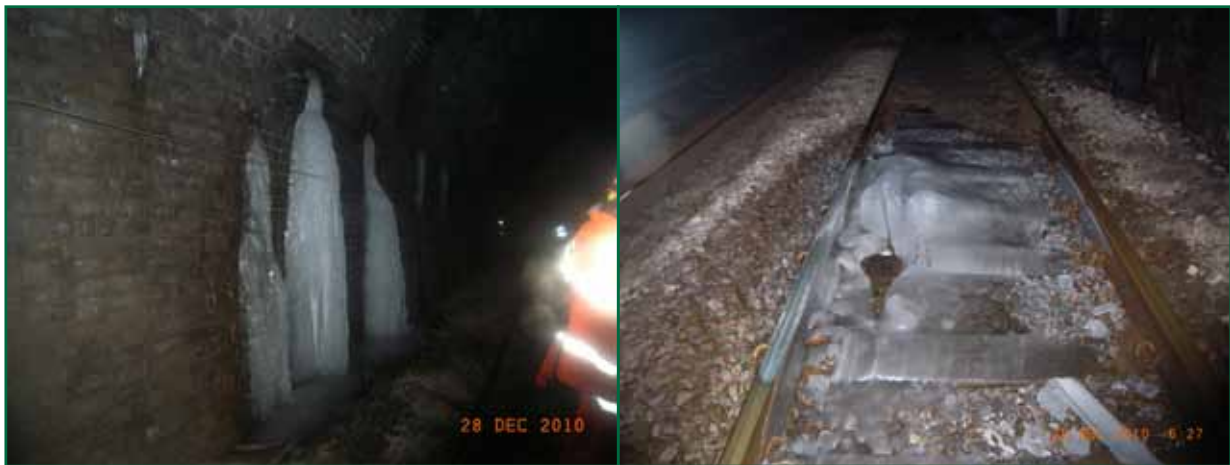
Figure 12: Ice formations found on the track and tunnel wall
